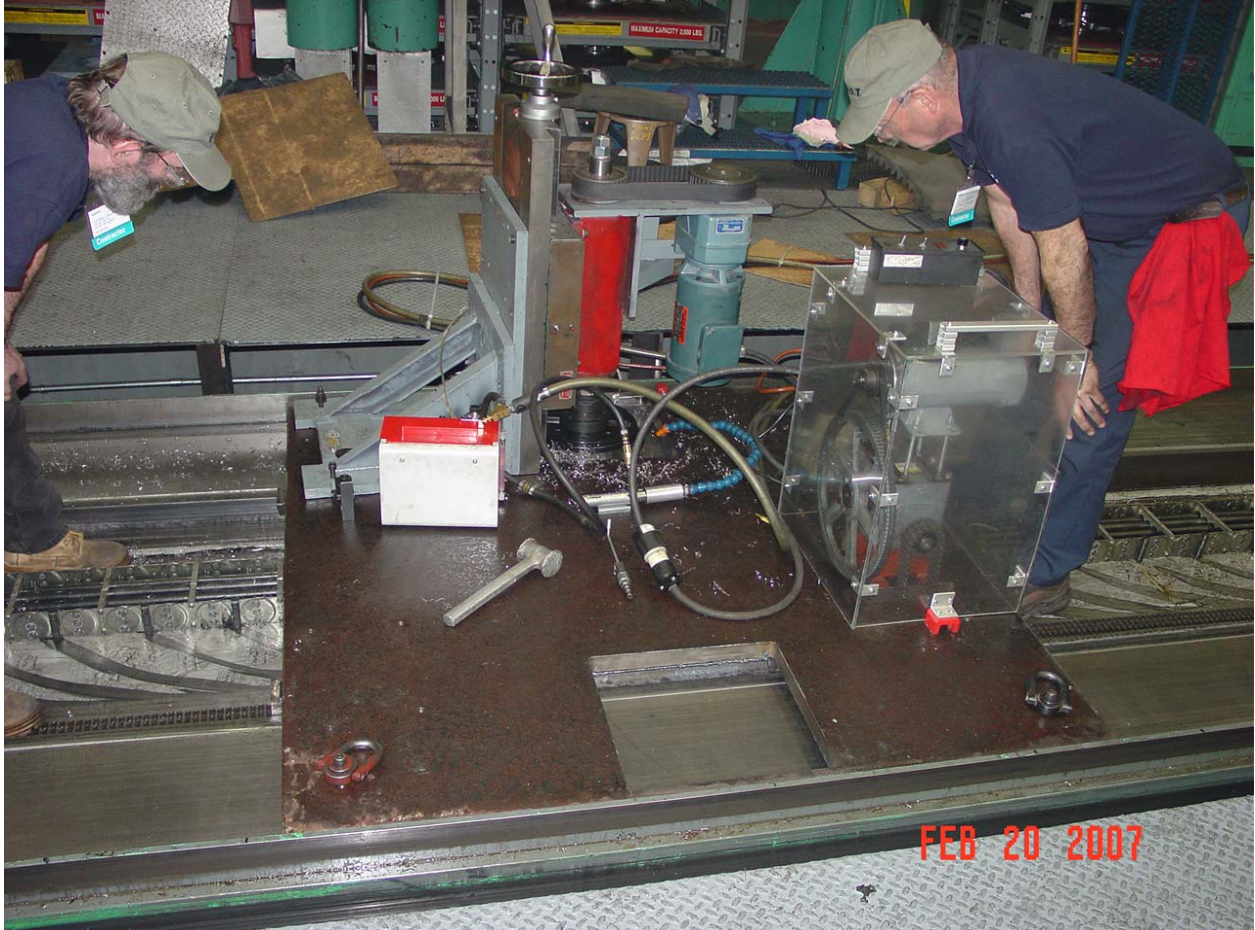
IMAGE 2. The temporary milling carriage, fit to accurate clearance surfaces with a moldable plain bearing material, with drive unit and milling spindle in operation. It was possible to carry a .002in deep cut for 140 feet.
